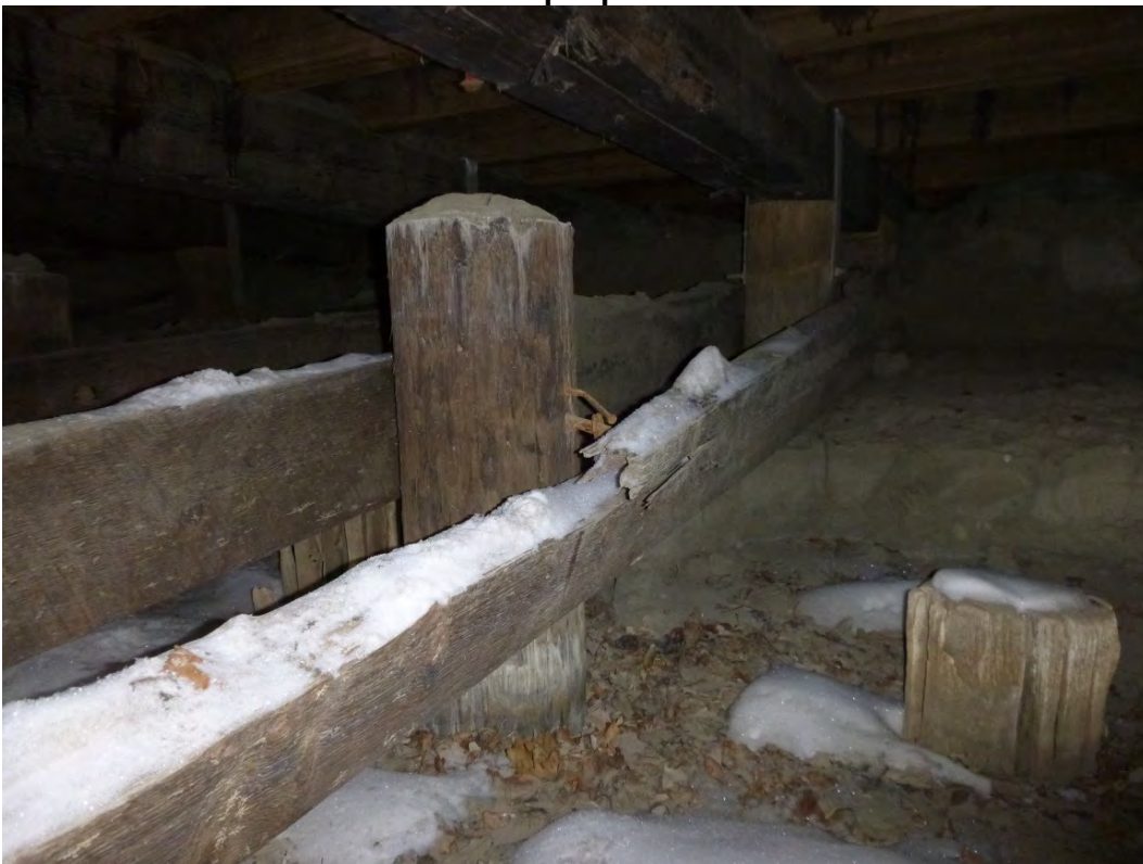
Photo 24 – Diagonal bracing member no long attached to pile
