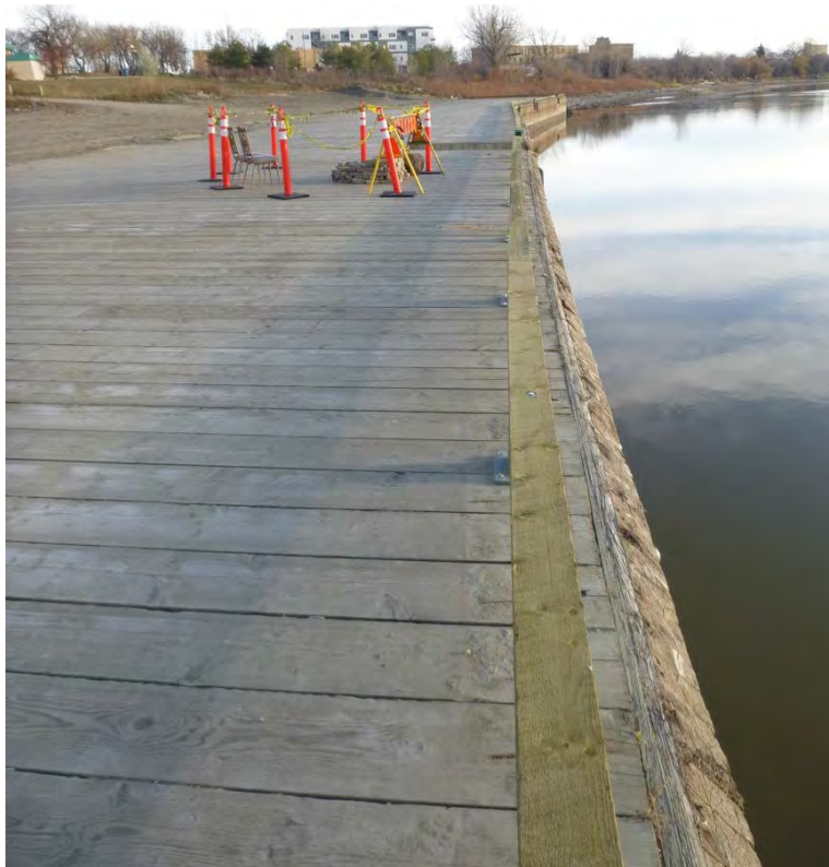
Photo 8 – Overall view of deck looking north; taken just north of South Slipway
