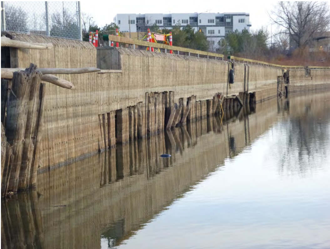
Photo 2 – East waterside skirting damage due to river ice erosion
