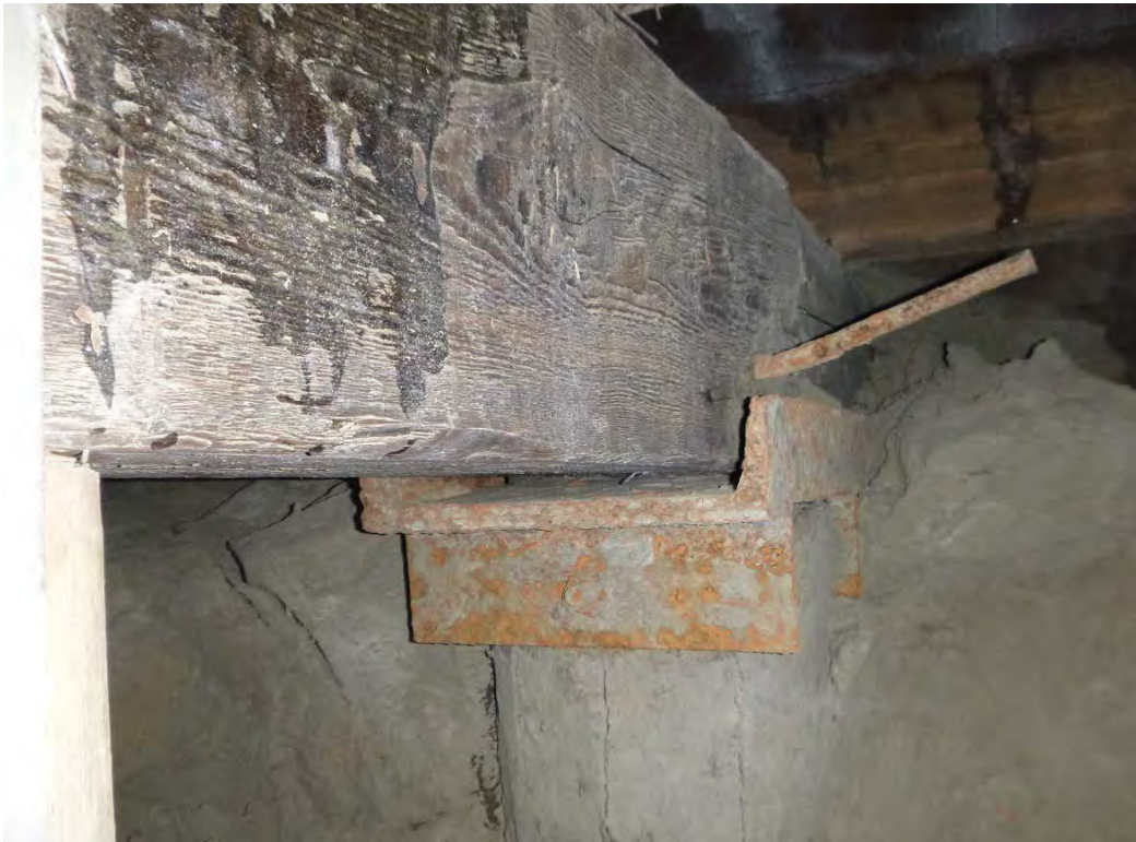
Photo 17 – Pile cap beam between E and C; reduced bearing length at steel seat
