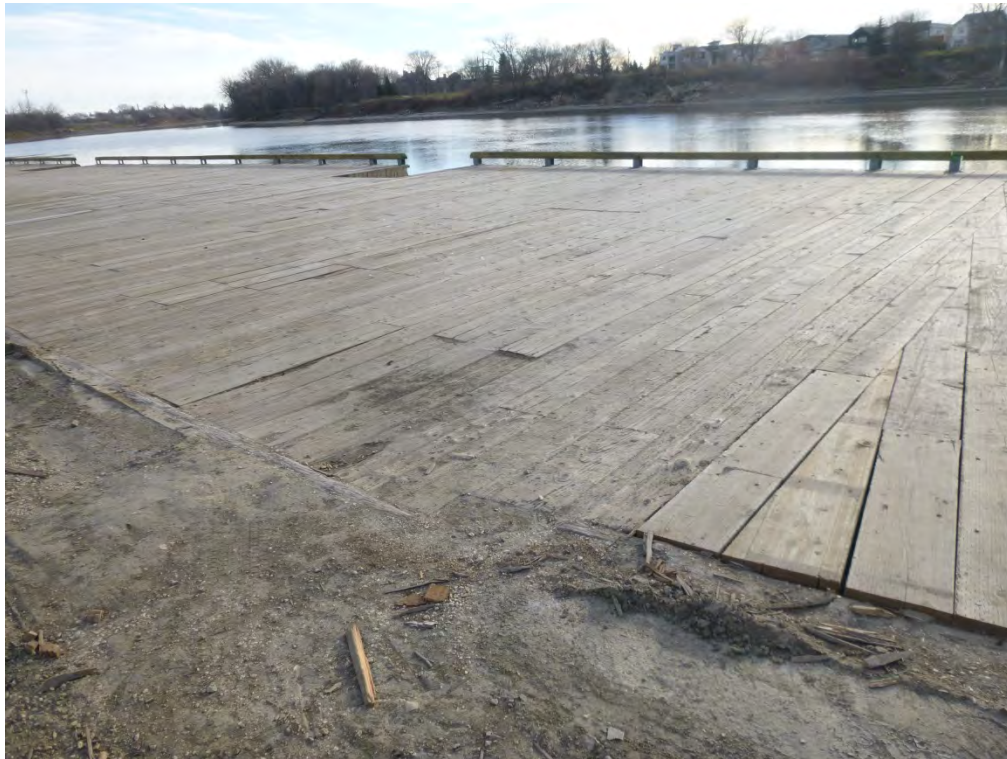
Photo 9 – Area of depressed and deteriorated planks opposite bend marking transition between Section 1 and Section 2, approximately 4.5 m in diameter
