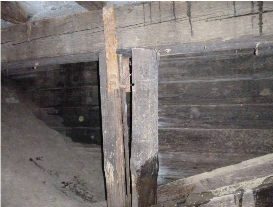
Photo 23 – Split pile at line 85
