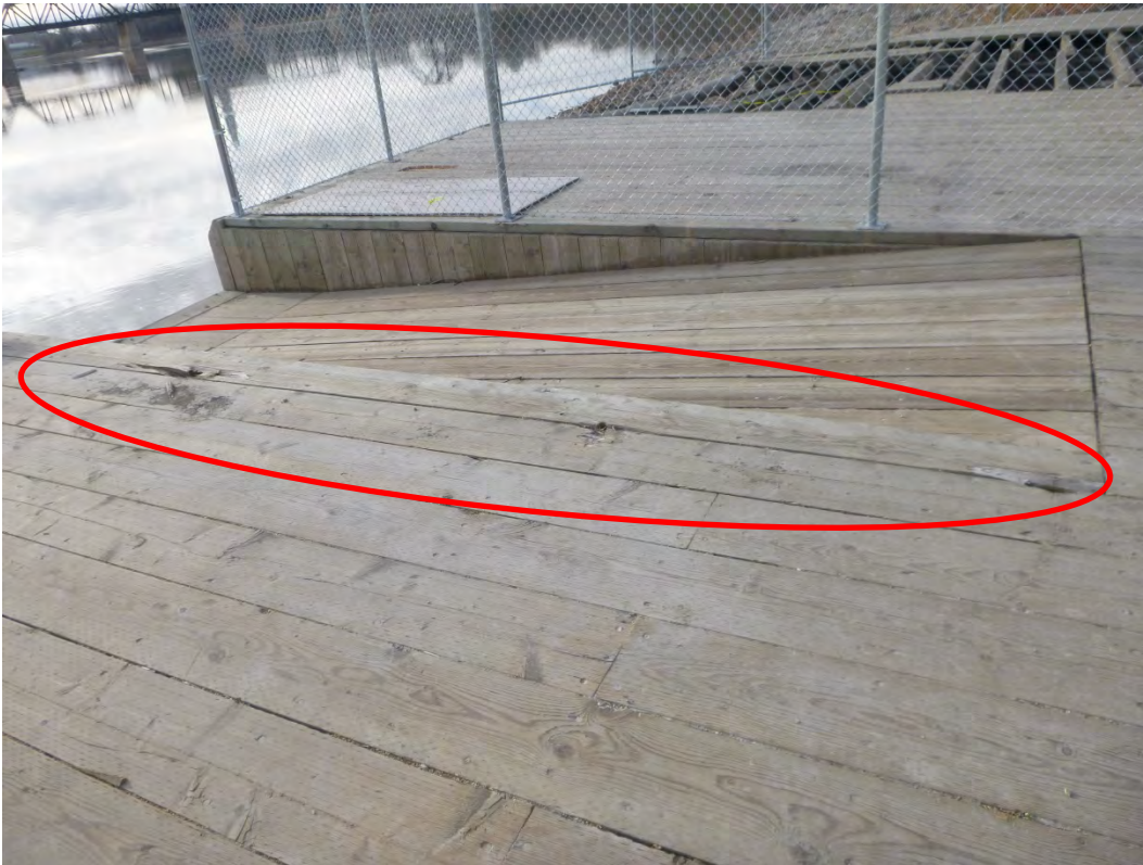
Photo 7 – Two planks adjacent to South slipway that require replacement
