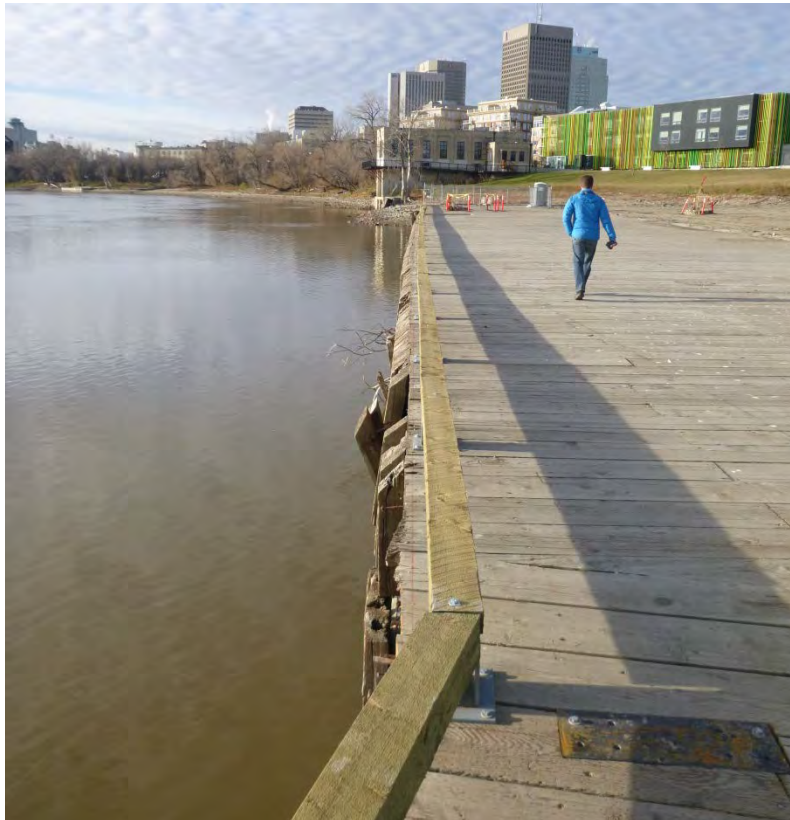
Photo 3 – Longitudinal view of Section 1 skirting showing horizontal deflection
