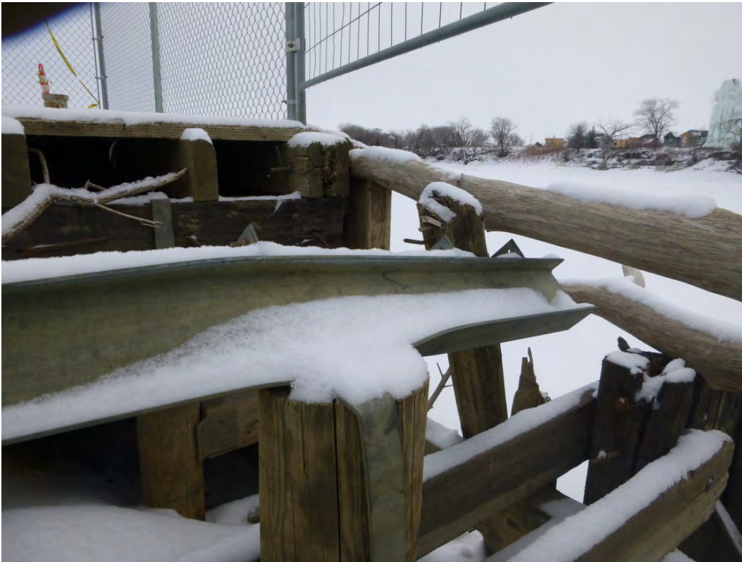
Photo 25 – Damaged upstream side of Alexander Dock
