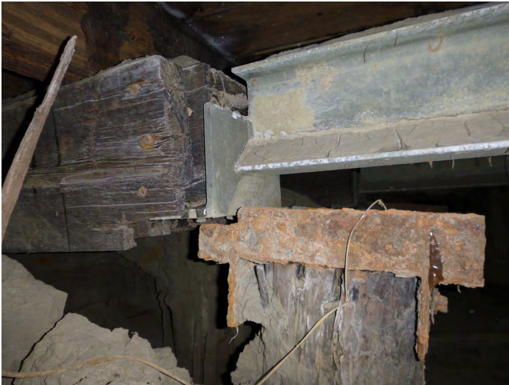
Photo 19 – Beam cantilevering out from riverbank and not bearing on pile, but supported on seat extension of steel beam. Beam has increased deterioration since the 2001 inspection.
