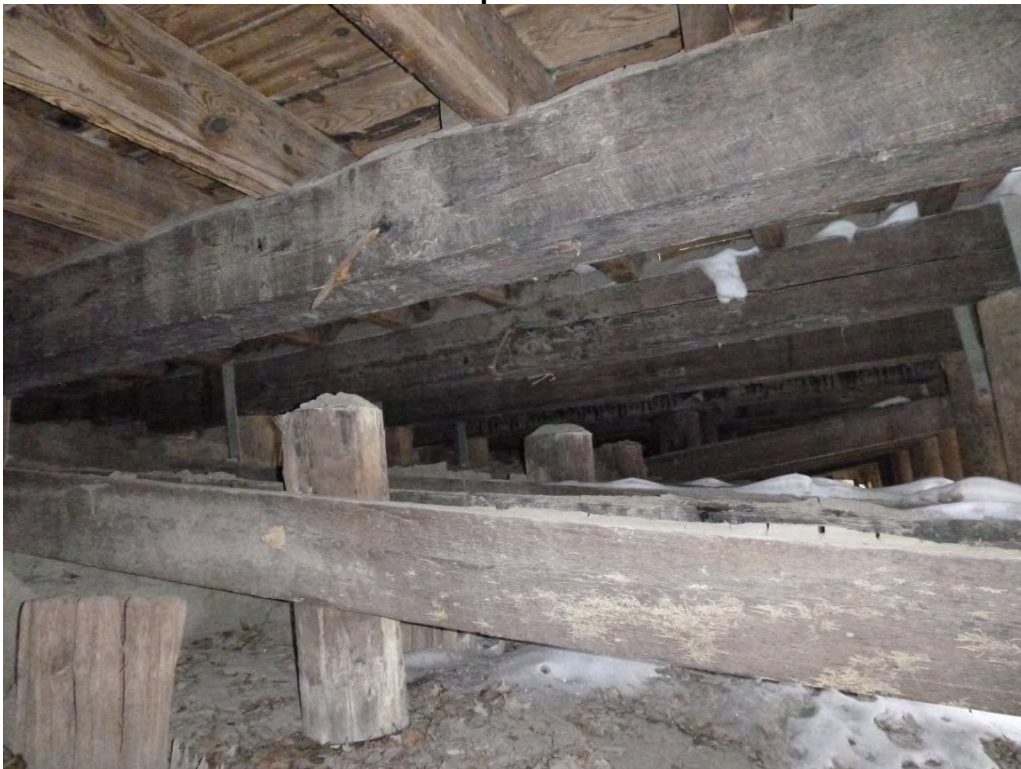
Photo 20 – Intermediate pier support shifted away from original timber pile cap beam
