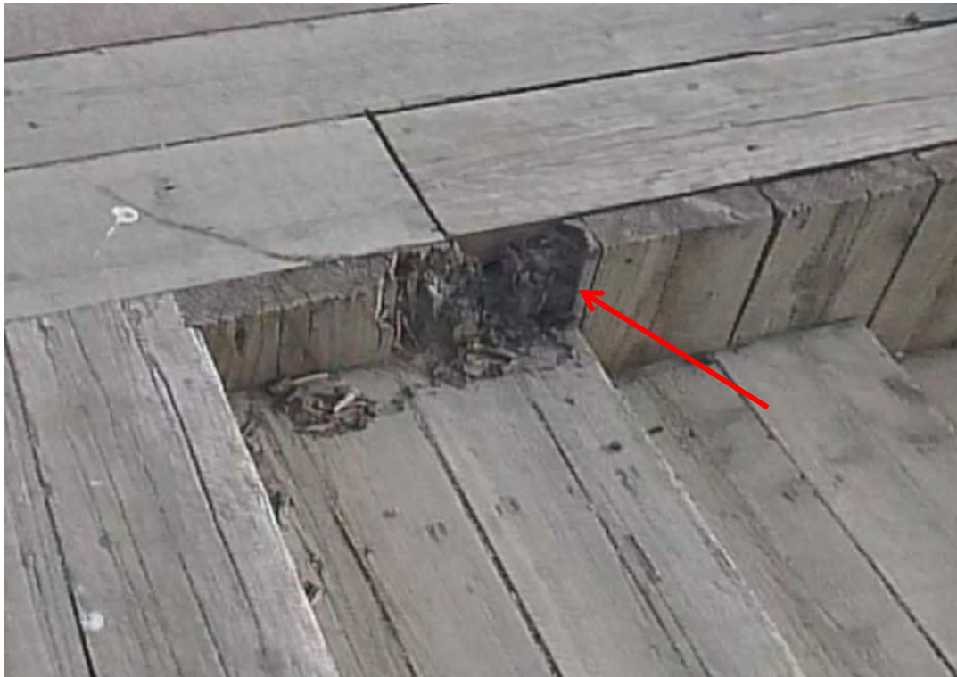
Photo 11 – Deteriorated plank at southern Section 2 slipway
