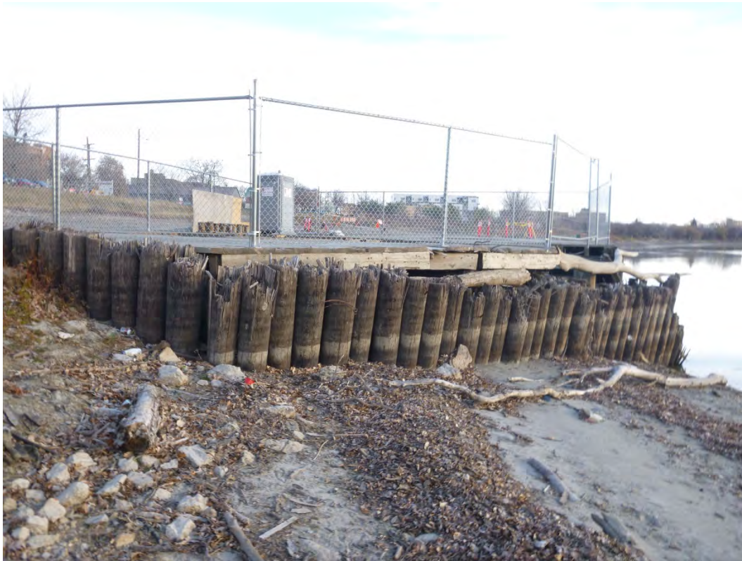
Photo 1 – South waterside skirting damage due to river ice
