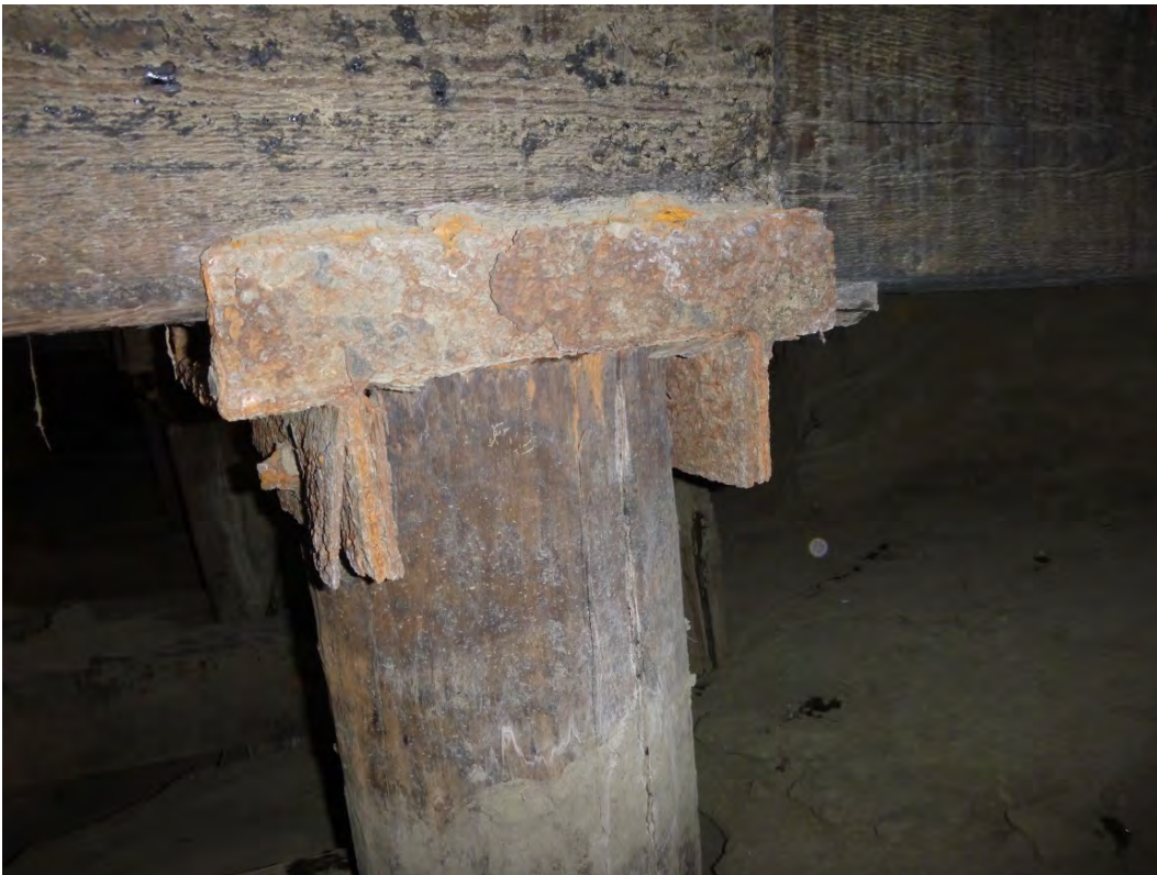
Photo 16 – Deteriorated steel pile cap beam support
