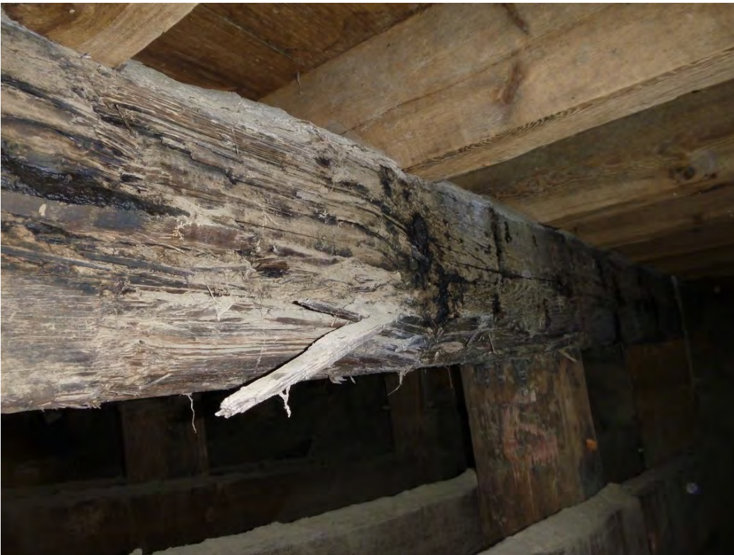
Photo 14 – Deteriorated pile cap beam at line 17
