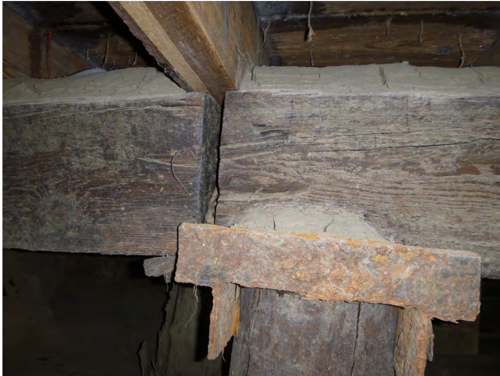
Photo 18 – Insufficient bearing length for beam cantilevering out of riverbank at pile along line C
