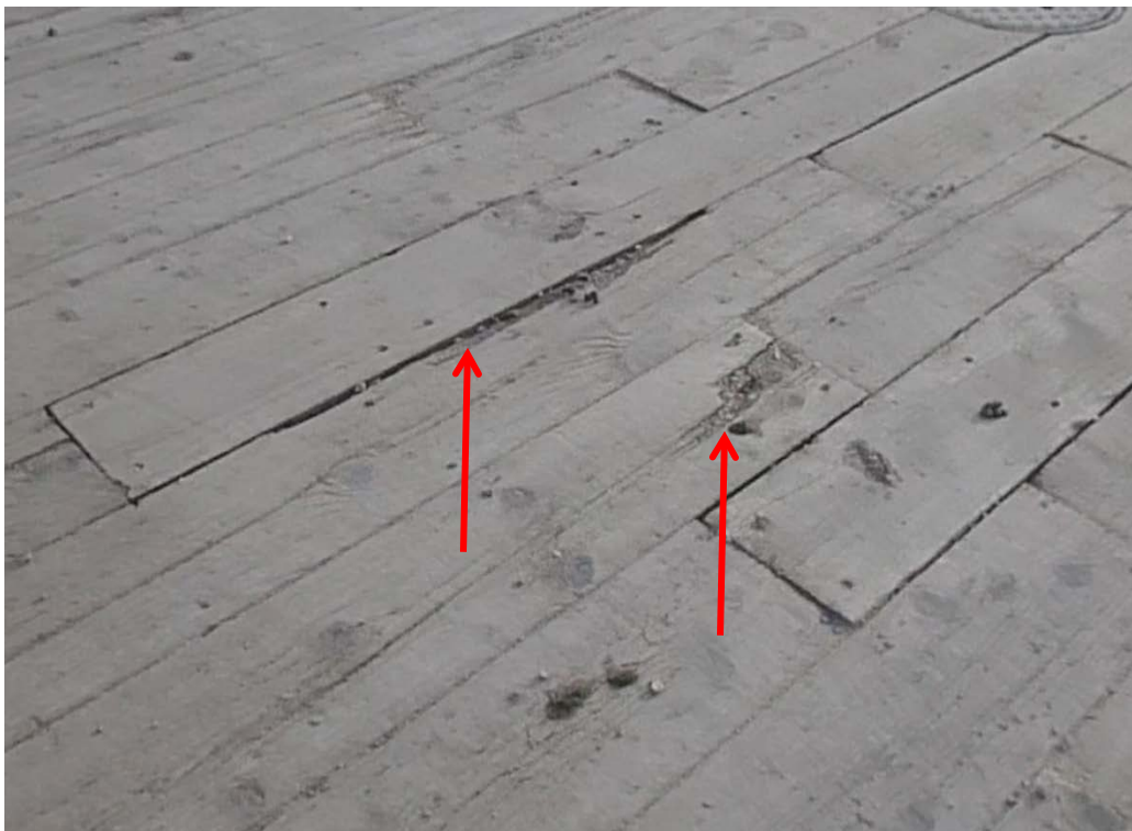
Photo 10 – Plank deterioration resulting in a trip hazard near the Section 1 / Section 2 transition
