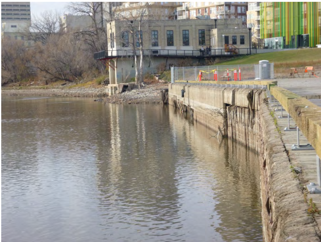
Photo 4 – View of deteriorated waterside skirting from the North end of Section 2
