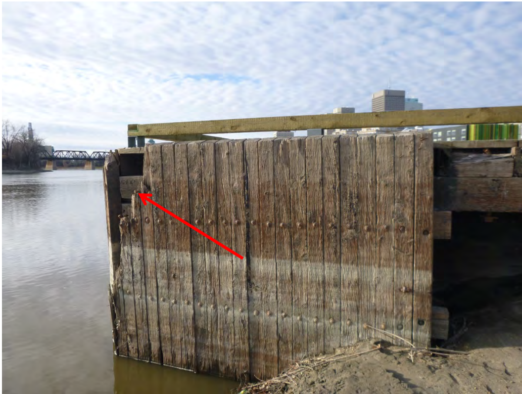
Photo 5 – North face of Section 2 with damage in upper left corner
